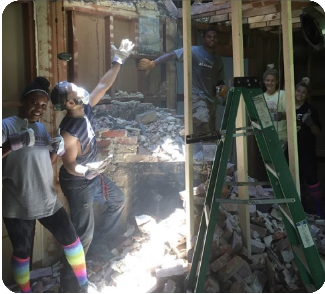
Abby Cisko is ready to take on any project with the help of her friends—like dismantling a fireplace, as shown here.
