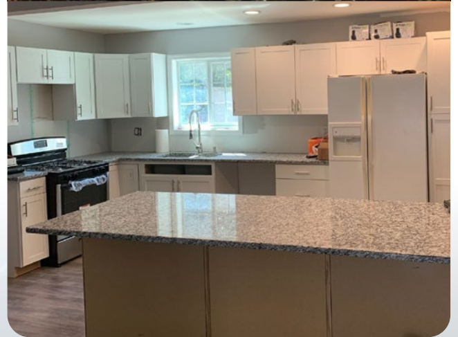
Top: A kitchen from House #2 in Flat Shoals, Georgia before (showing fire damage) Bottom: Kitchen after remodel.
